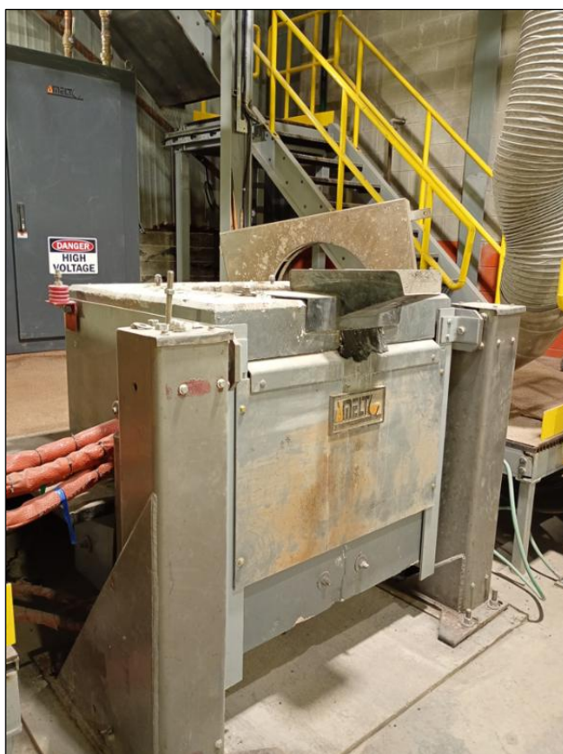
Photo 19.2-1 Photograph within the gold furnace room taken while on site visit 8 October 2025.
